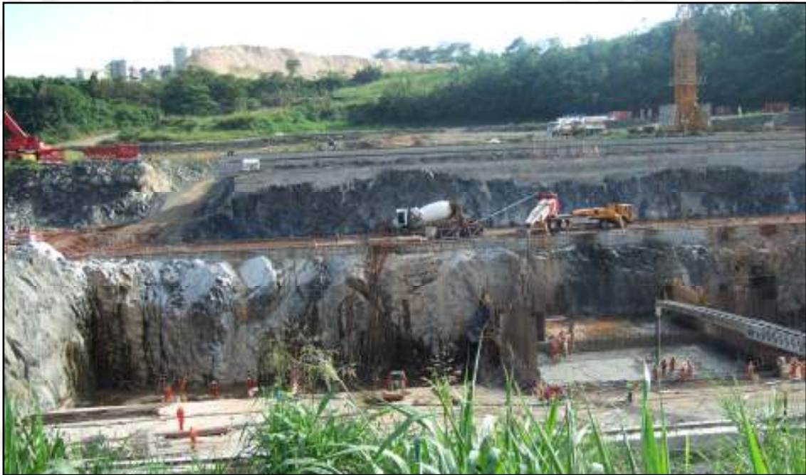
Construction of the Powerhouse Emerges Out of the West Channel River Bed - October 2008
