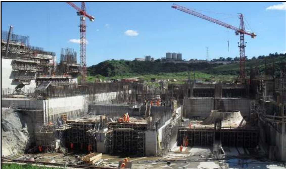
A Year Later the Powerhouse with the Turbine Housings Being Constructed - October 2009
